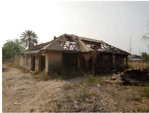
Some destroyed houses at Tudun Adabu
